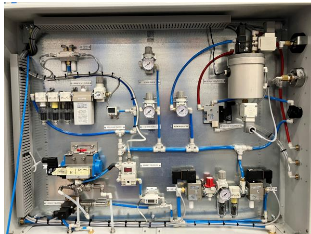
Figure 3 - Pneumatics / hydraulics cabinet
